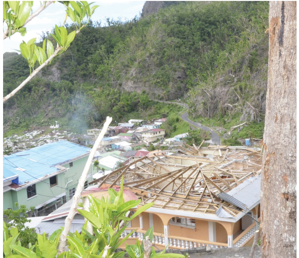
Most roofs were damaged or destroyed in the storm. Flickr photo by The Commonwealth, https://www.flickr.com/photos/comsec/
