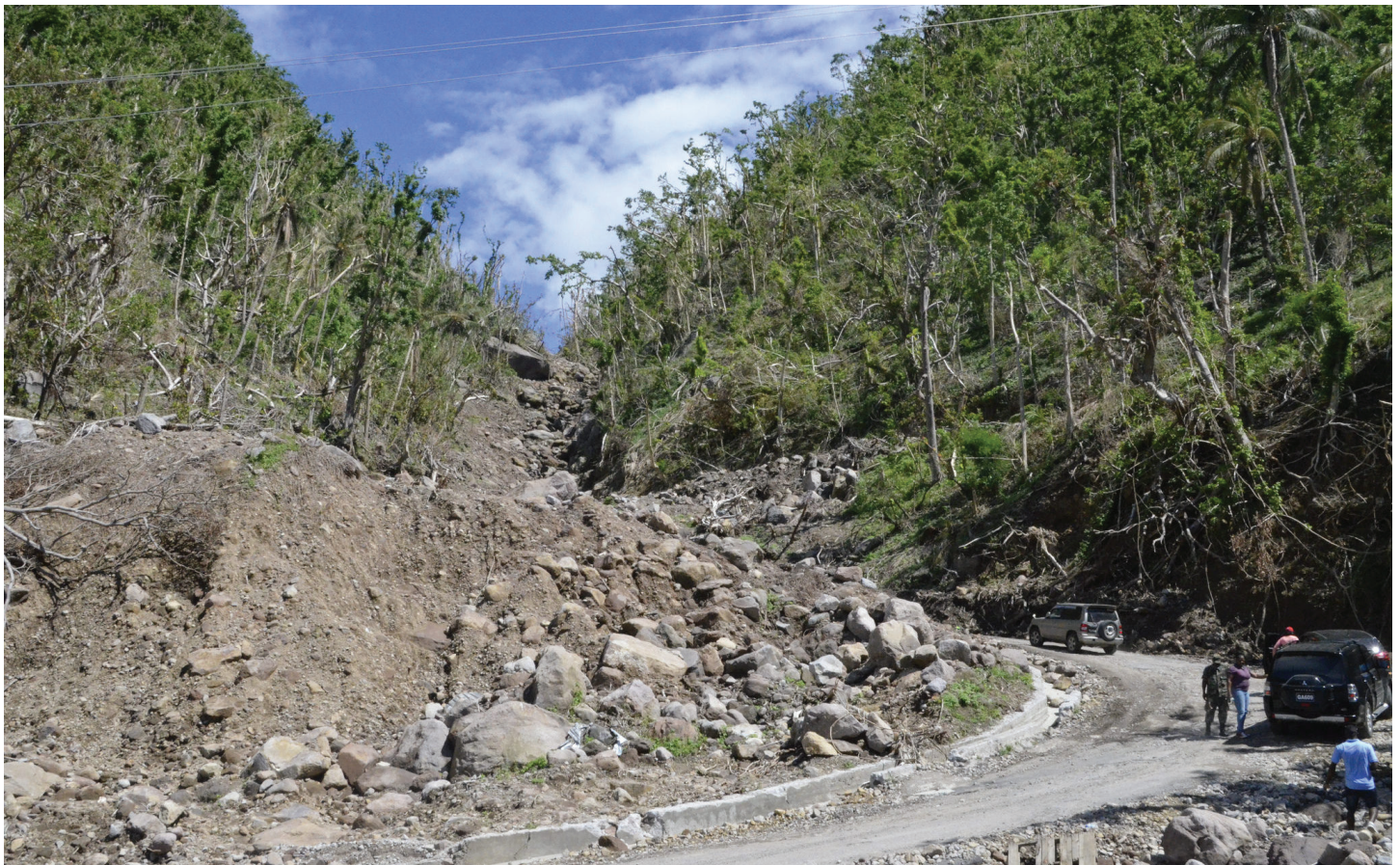
Many of Dominica's roads were heavily damaged by the recent hurricane. Flickr photo by The Commonwealth, https://www.flickr.com/photos/comsec/
